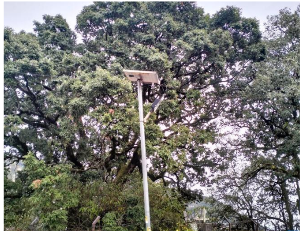
Solar Street Light
